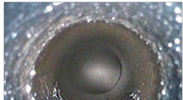
Supply tube view from the locating flange area towards the elbow transition
